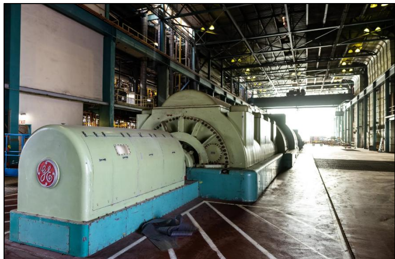
Unit 2, one of the two original 1950s-era General Electric gas steam generators cooled with Pacific Ocean water and set to be phased out by 2029 at the Scattergood Generating Station in Los Angeles, March 17, 2022.
